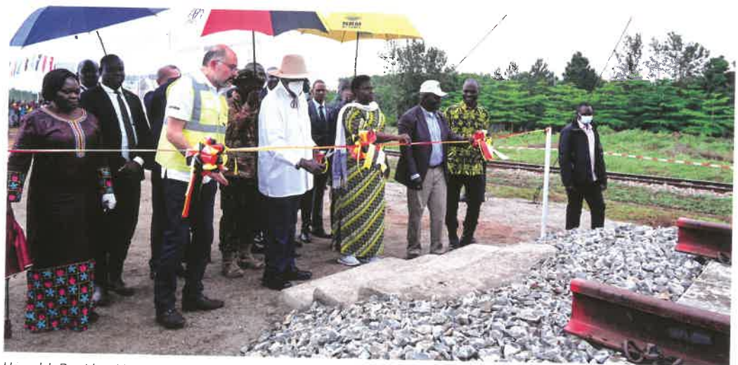
Uganda's President Yoweri Museveni launched construction of that country's 272 km Eastern Line from the capital Kampala to Malaba on the Kenyan border with a ceremony in Tororo district on November 21. A €2.7bn contract to build the line had been awarded to Turkish contractor Yapı Merkezi on October 14 (RG 12.24 p9).
